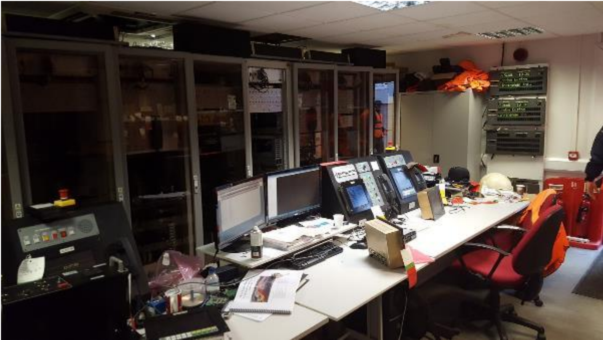
Figure 8.1: Alstom's TMS simulator at Oxley Depot
